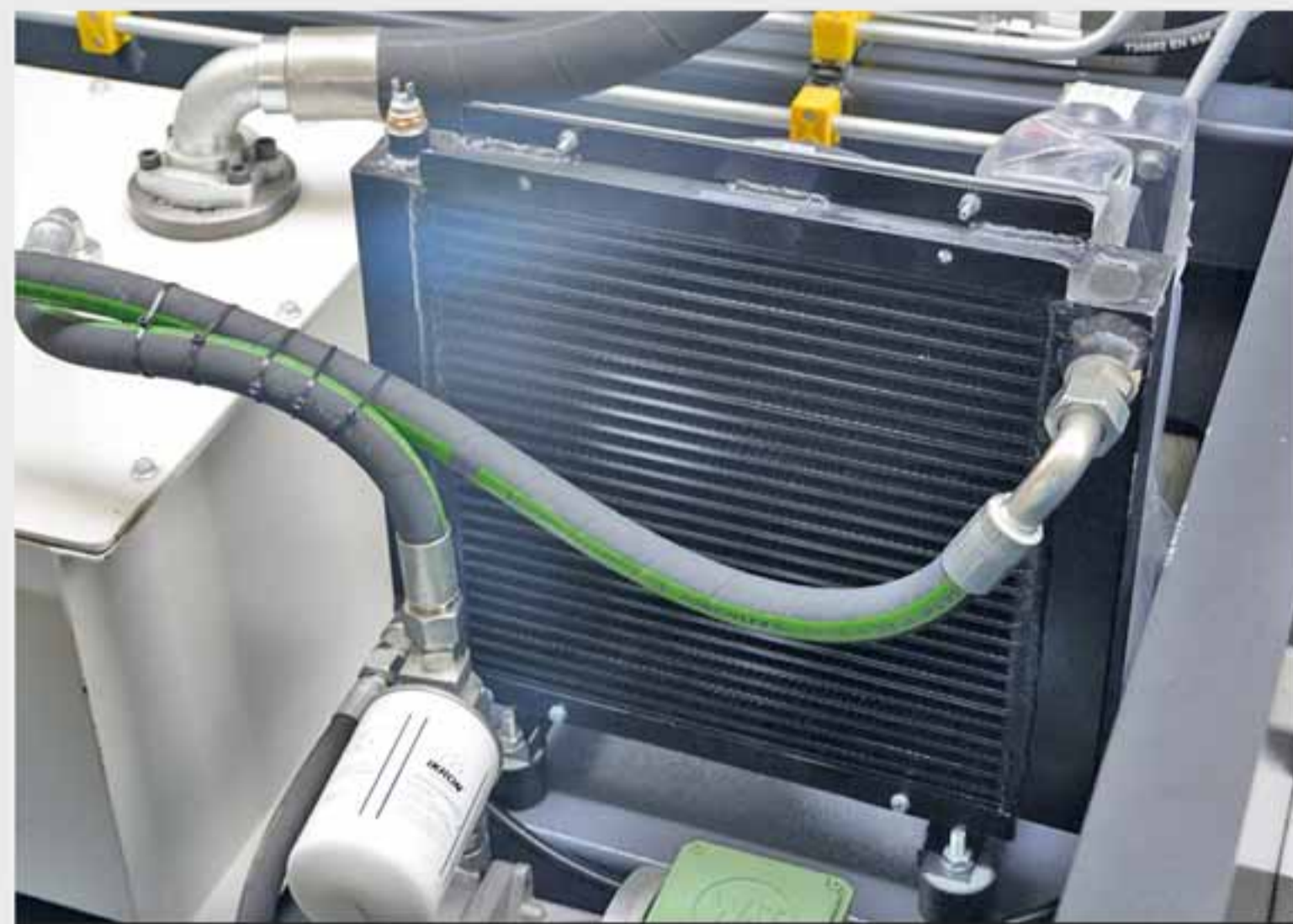
Hydraulic Oil Cooling Fan System Heater For Oil Tank
